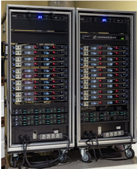
The racks contain 21 EM 6000 Dante receivers as well as a L 6000 chargers for the mini bodypack transmitters
